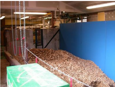
Wood chip heating system at Weathersfield School.
