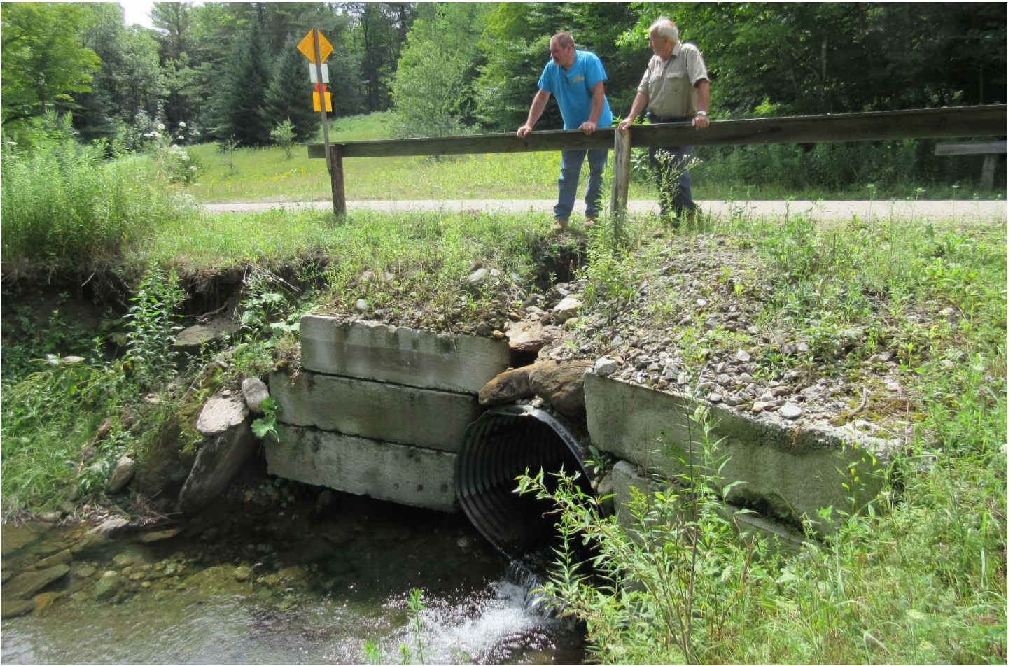
Top: Downstream end of culvert. Culvert and headers are undercutting. Cover above the culvert is destabilizing at the edge of the roadway. August 2, 2016
