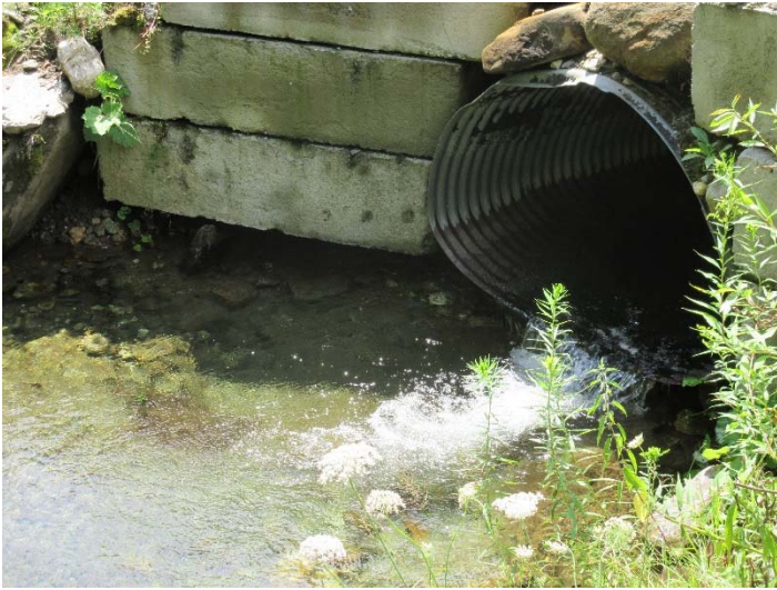
Top left: Undercutting of culvert and headers.
