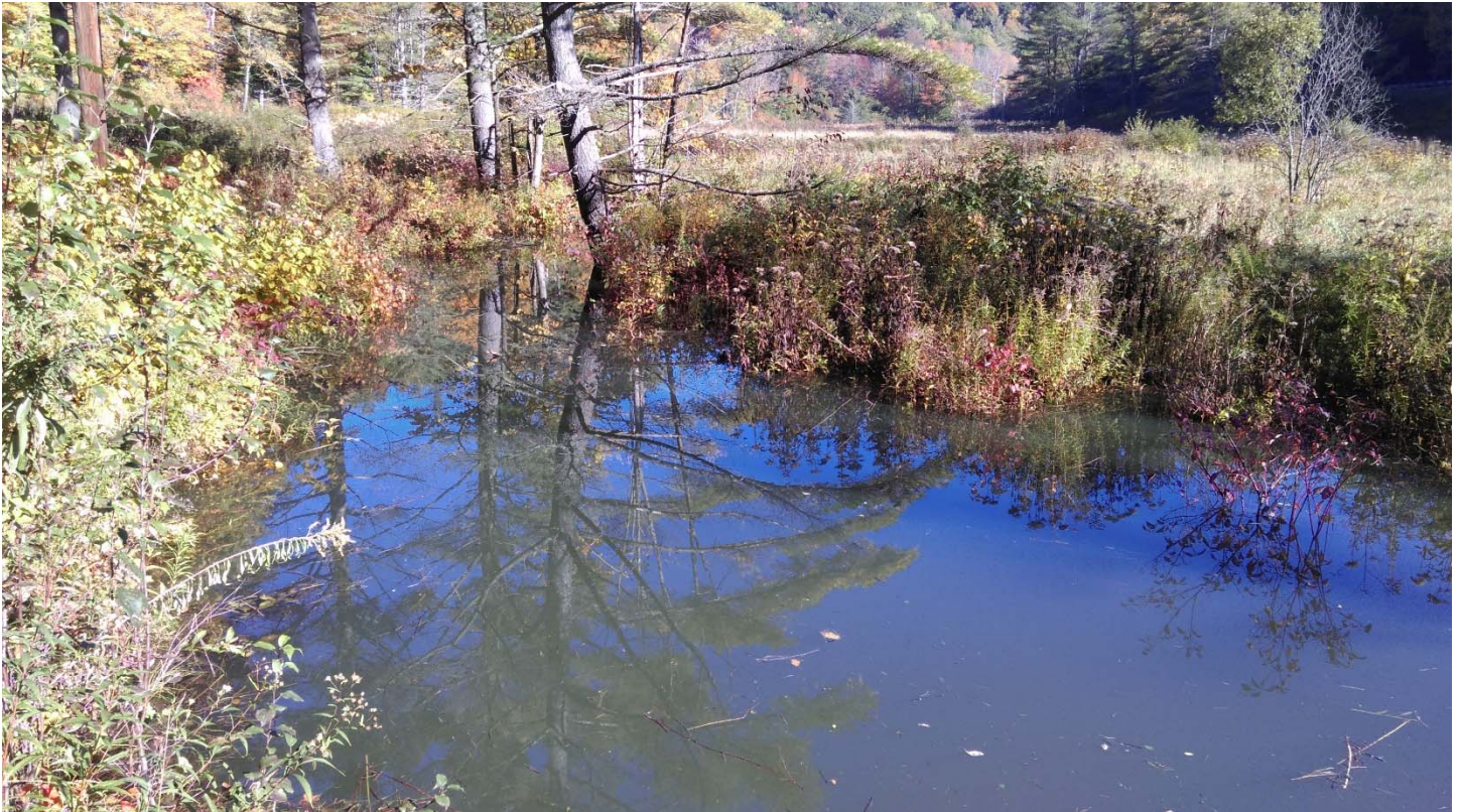
Bottom: Water trapped in adjacent wetland upstream from culvert blocked by beaver dam.
