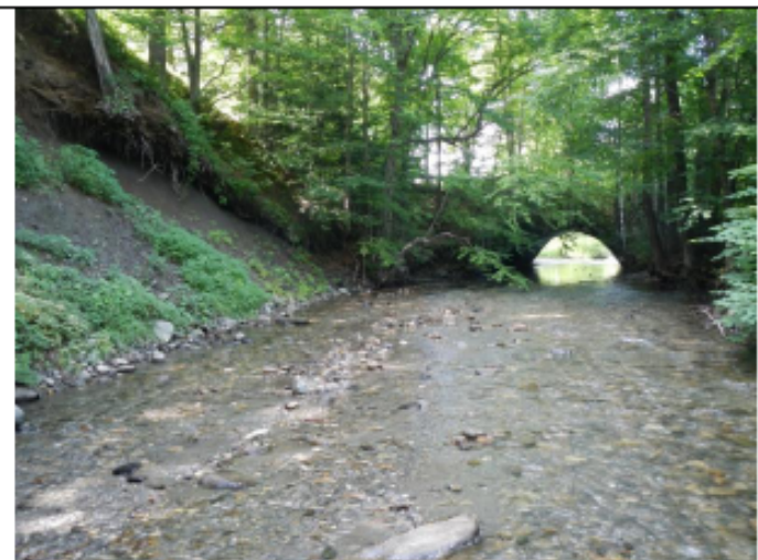
Undersized arch and downstream mass failure
