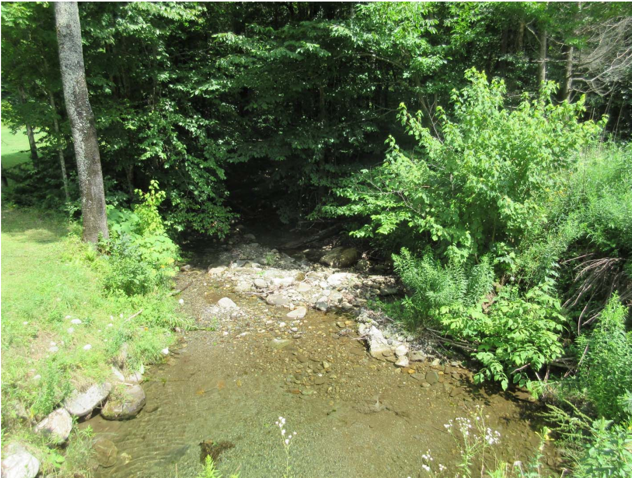
Top: Looking downstream from the culvert. Plunge pool is in the foreground and then the stream narrows up.
