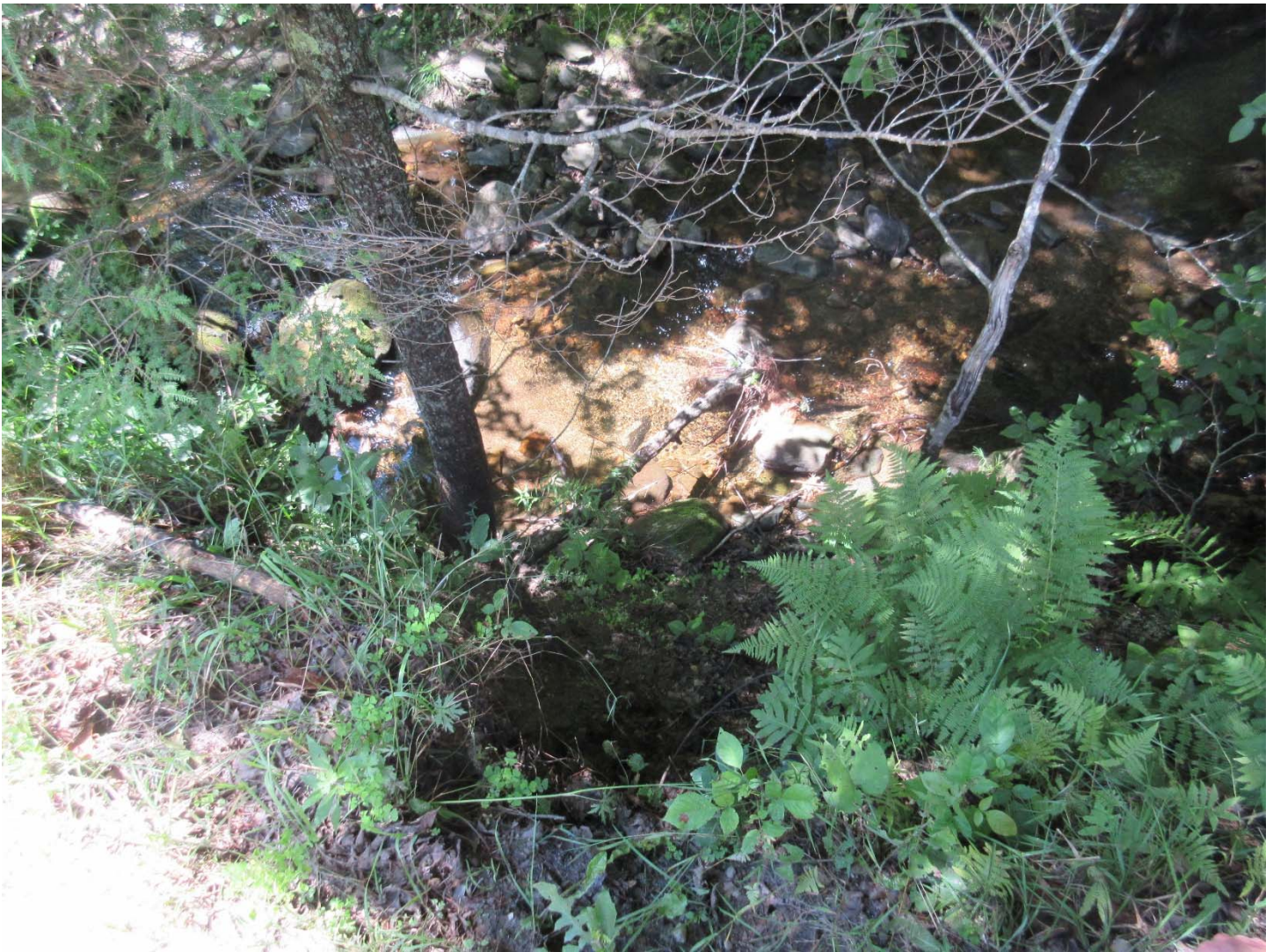
All: Bank destabilizing where trees stop.
