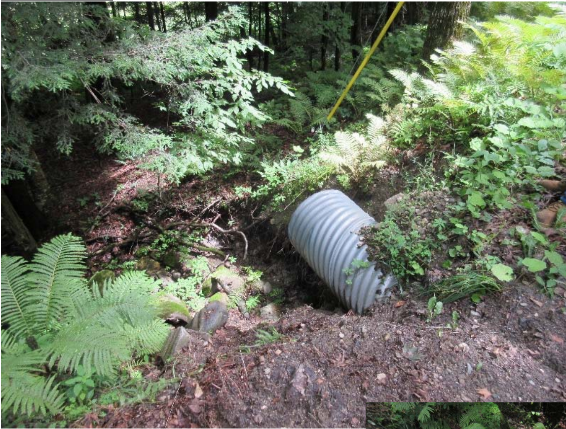
Top left and bottom left: Road material flowing into stream next to culvert
