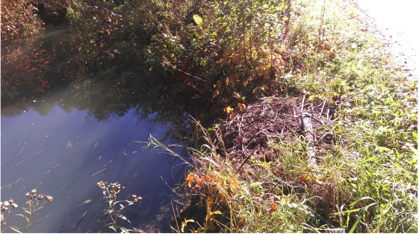
Top: Beaver dam blocking the culvert entrance with water trapped in adjacent wetland.
