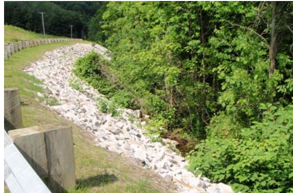
Figure 9. Rip-rap on the left bank of reach T2.01 along State Farm Road
