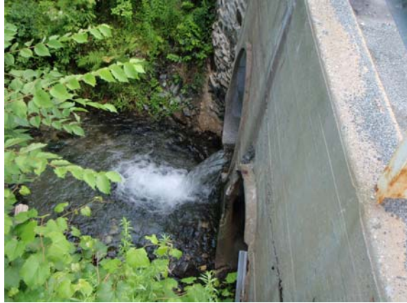
Figure 8. Perched culvert at the State Farm Road Crossing
