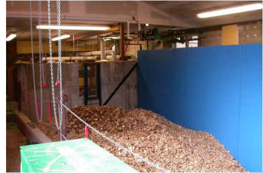
Figure 27: Wood chip heating system at Weathersfield School.
