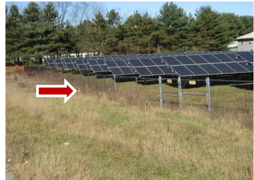
Figure 24: This project is an example of inadequate landscaping/screening. Note deciduous shrubs do not provide year-round screening, small plants will take many years to grow up to provide effective screening, and a lack of mowing the grass between the landscaping and roadway, which is to the left of the photo.
